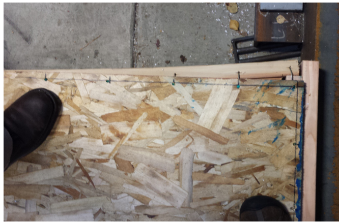
Figure 14. A typical failure mode at boundary framing of Part A diaphragms.
